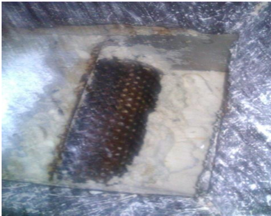
Figure A10: Grating surface rusting with time
