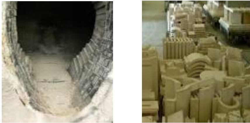
Figure 2. 3 (a) Furnace refractory (b) Different types of refractory shapes
