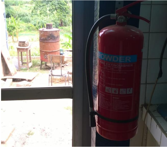
Figure 3. 6 Fire extinguisher close to the firing area.
