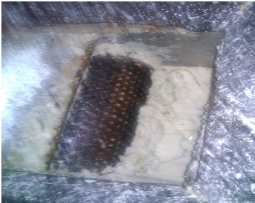
Figure A10: Grating surface rusting with time
